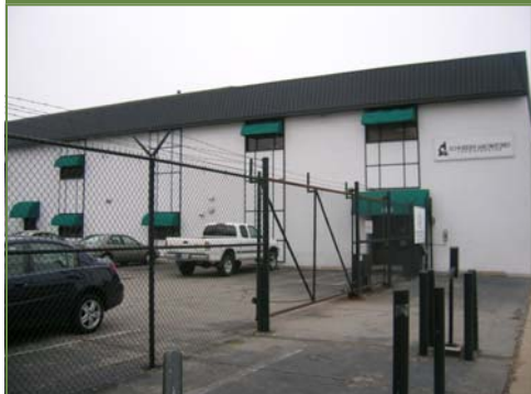
Chain-link fencing with barbed wire on West Cary Street are not appropriate fencing materials
