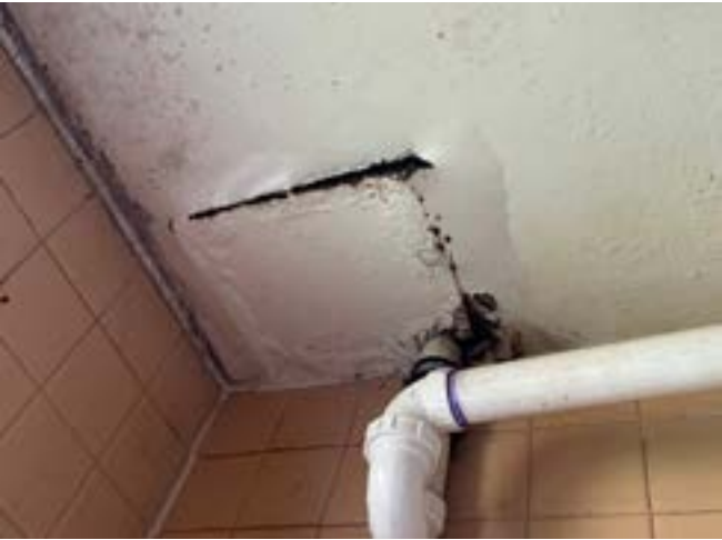
Lack of ventilation creates bathroom ceiling issues.
