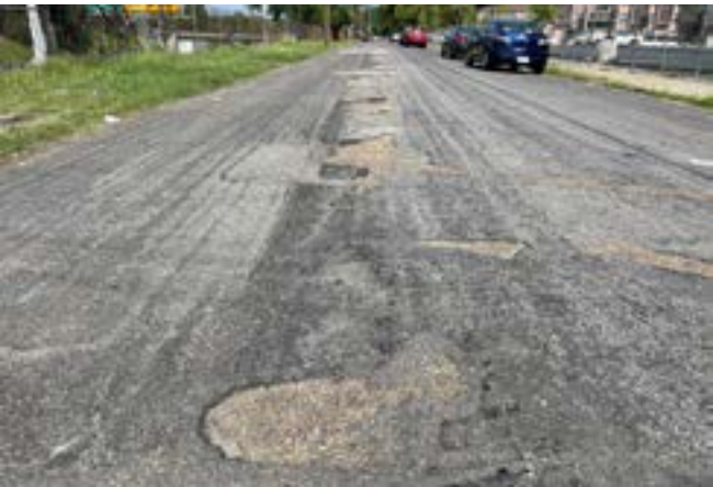
Streets in North Jackson Ward around Gilpin Court are in need of infrastructure updates.
