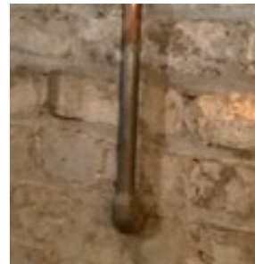
Horizontal pipe between wall and first pipe bend/fitting is not visible. Still submit photos of a scratch/magnet test for the portion that is visible.
