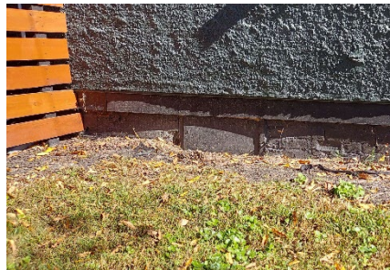
Crawlspace is too narrow to enter.
