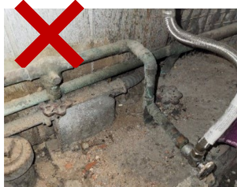
Shows multiple pipes without labels, and the scratch/magnet test is not visible
