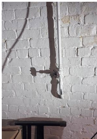
Photo 1: Close-up of scratch & magnet test and point of pipe entry from the ground or wall
