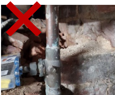
Does not show the entry point of the pipe into the building and a scratch/magnet test
