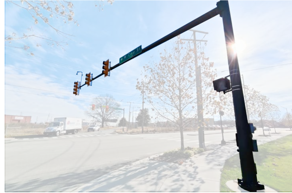
Traffic light signal poles are designed to match the site furnishings through the project, including color and detailing.
