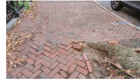
Large street trees have uprooted brick pavers
