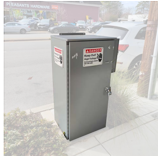
Utilities located along in streets are inadequately screened from the road or sidewalk.
