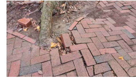
Uprooted brick pavers from tree roots
