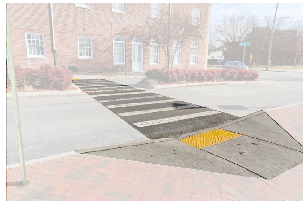
Pedestrian crossings are currently a CG-12 ramp and white block style painted asphalt.
