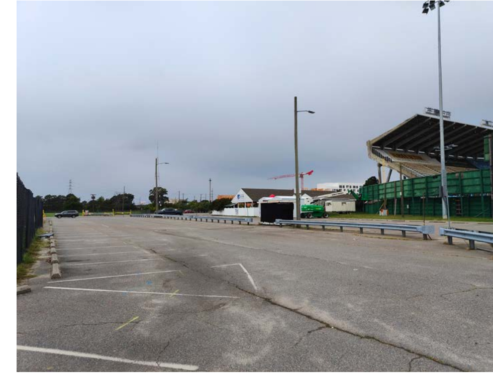
Existing parking lots are in poor condition.
