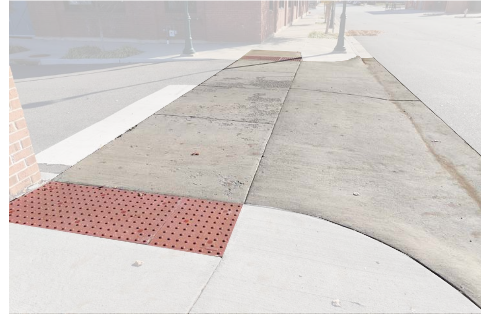
Concrete is used for aprons through the Sauer project, offering a different material for pedestrian crossings, and speed of road delineation.
