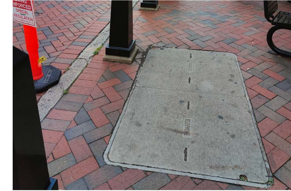
Manholes and utilities are located in the center of the sidewalks for quick access, but do not blend with the surrounding materials.
