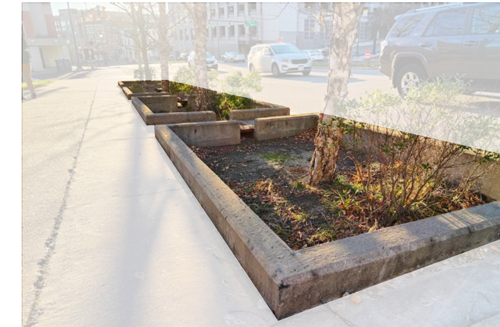
Tree wells located along 14th street are designed for stormwater capture, yet poor design and maintenance results in dangerous element for pedestrian users.
