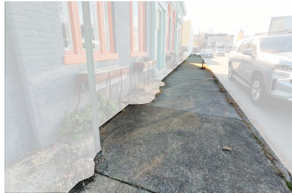
A lack of street trees and delineation from the Frontage Zone and the Pedestrian Travel Zone on side streets results in a poor streetscape.
