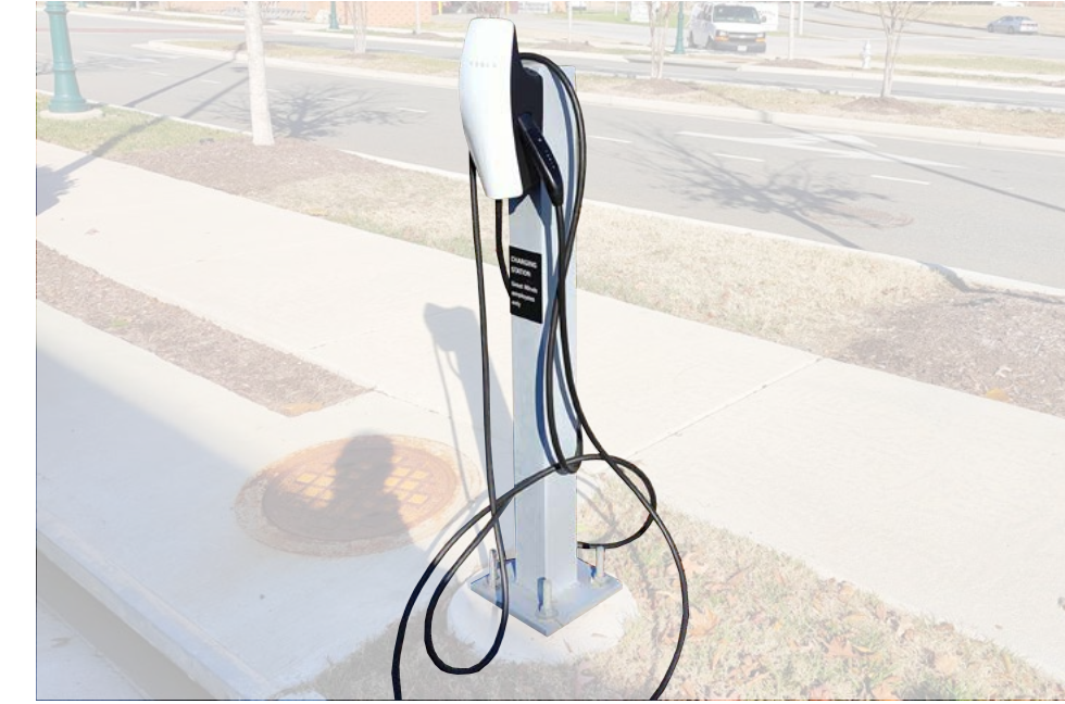
Electric car charging stations are provided throughout the project, increasing the likelihood of users to the site.
