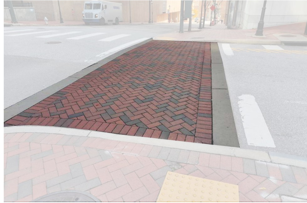
Pedestrian crossings include a concrete border and a herringbone brick paver pattern.
