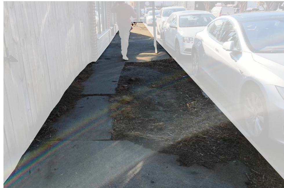
Poor maintenance has resulted in spreading mulch beds, cracked mossy sidewalks, and weed growth.
