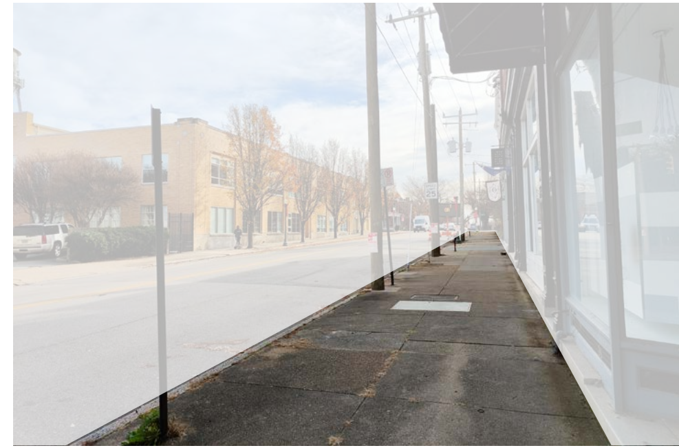
A lack of maintenance has caused Church Hill sidewalks to have cracks, moss, and weed growth.
