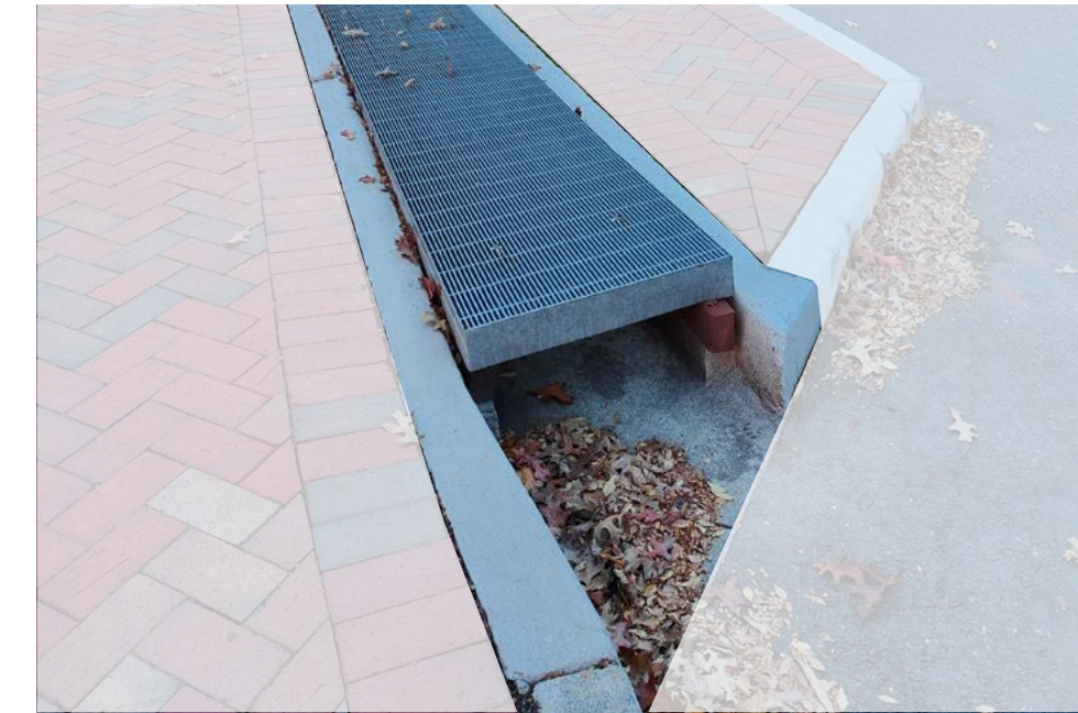
Storm drains are decorative metal which offers visual variety from the typical Richmond storm drain.
