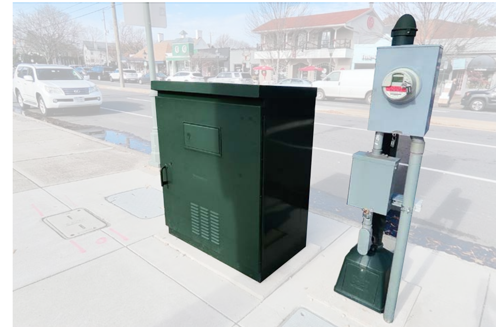
Utilities along the road are not screened, and obstruct users of the sidewalk.
