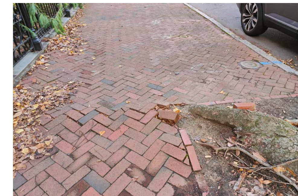
A lack of maintenance has caused tripping hazards and a poor surface for wheelchair users.
