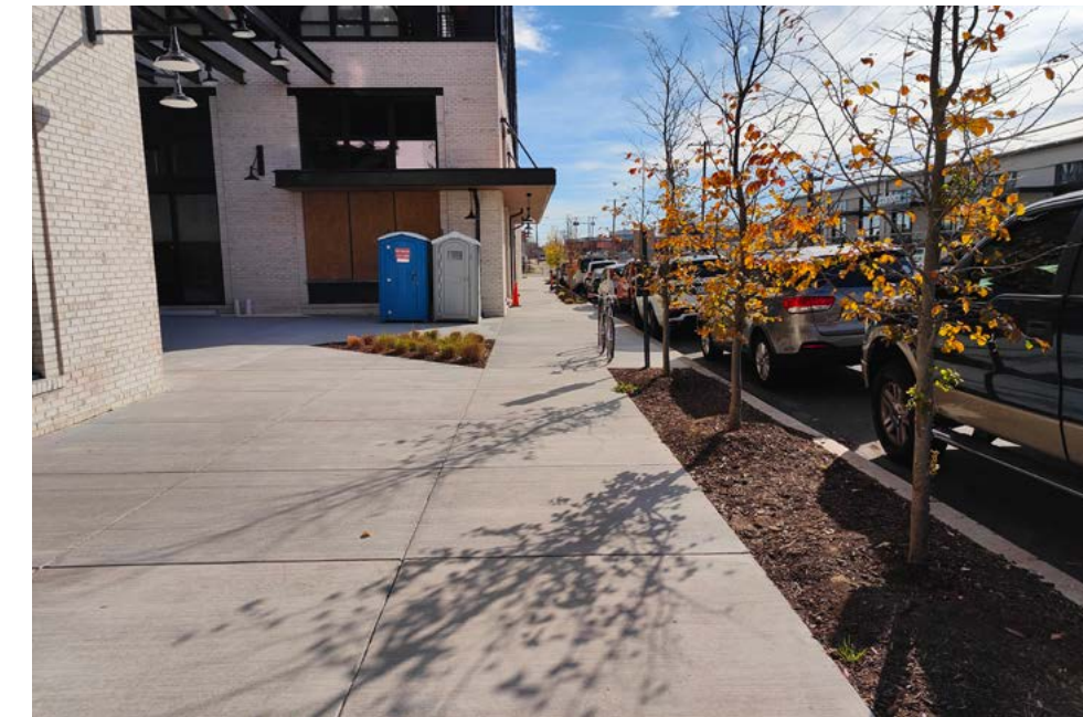
Difficult to identify public and private property from a lack of material diversity.
