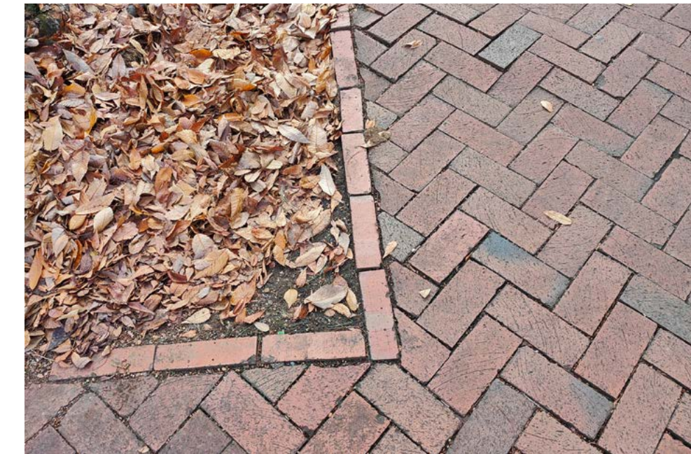
Brick pavers are used in multiple places throughout the streets, including borders, accent bands, and main thoroughfare routes.
