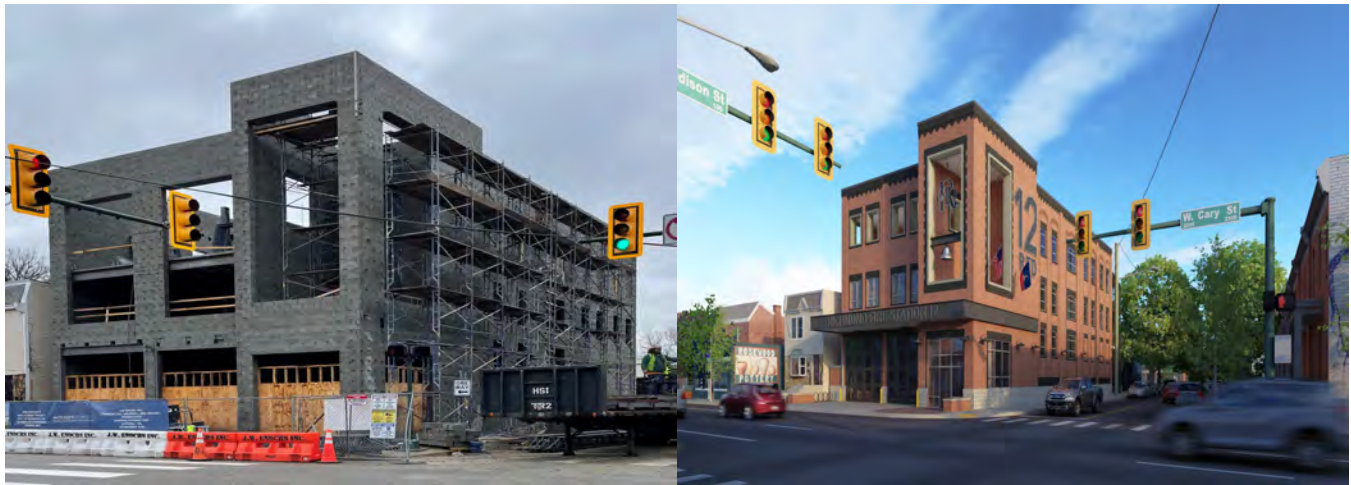
Left: Construction of Fire Station 12, as of December 29, 2023. Right: Rendering of completed building.
