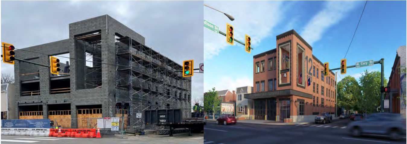
Left: Construction of Fire Station 12, as of December 29, 2023. Right: Rendering of completed building.
