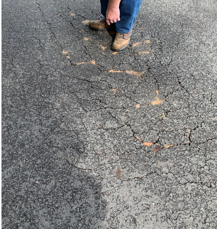
Alligator cracking with mud
