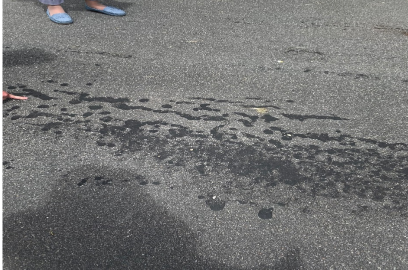
More bleeding pavement
