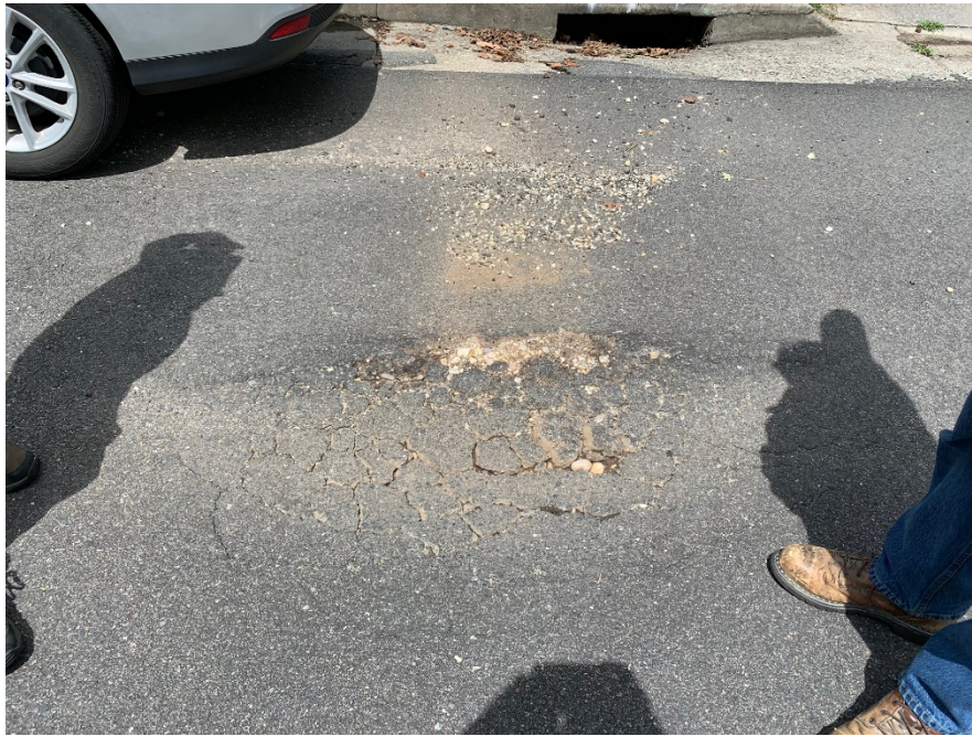
Cracking and depression with exposed dirt and river rock
