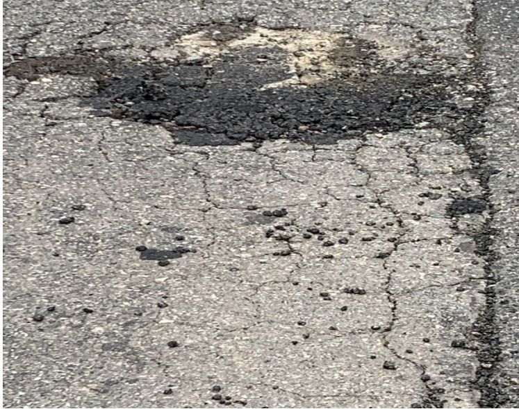
Cracking among the patch
