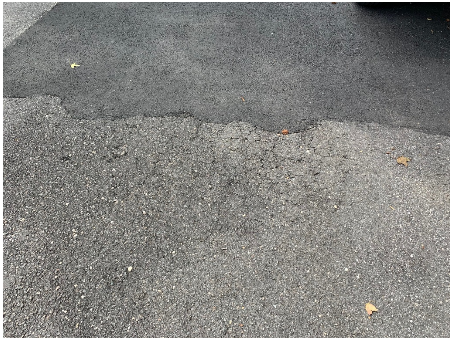
Cracking and patching
