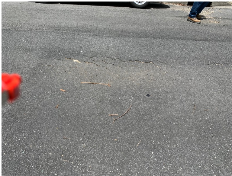
Cracking and depression in road
