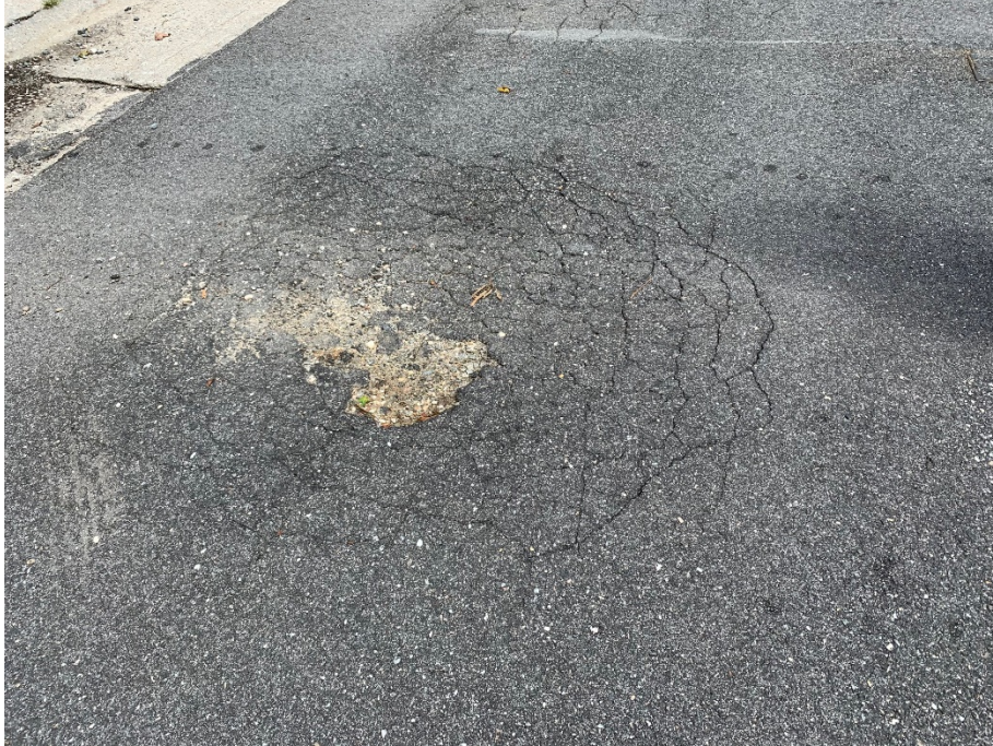
Cracking and pot hole with exposed dirt and stone
