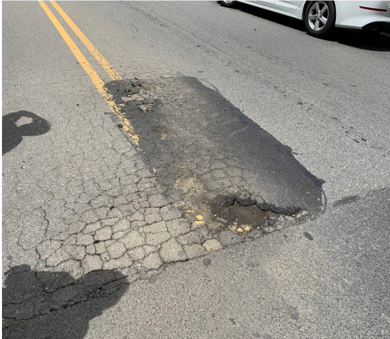
Cracking patch unraveling
