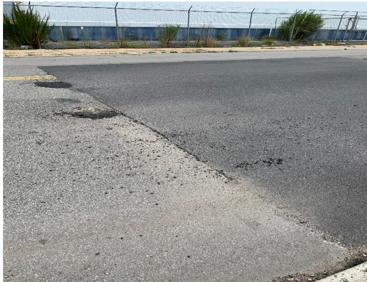
Patch appears to be falling apart
