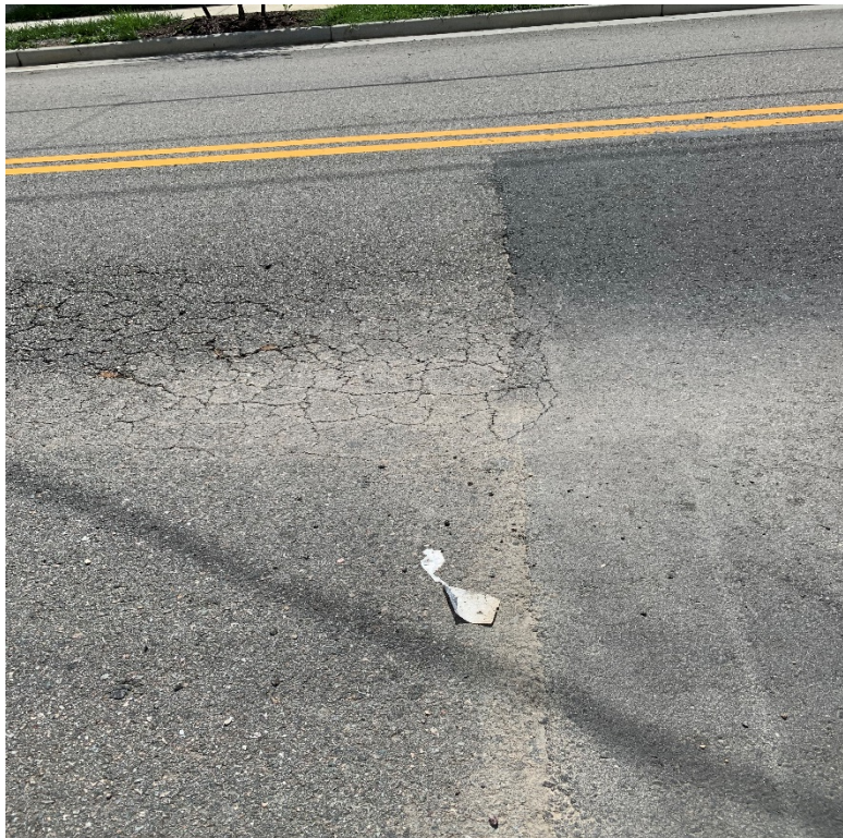
Cracking around a patch
