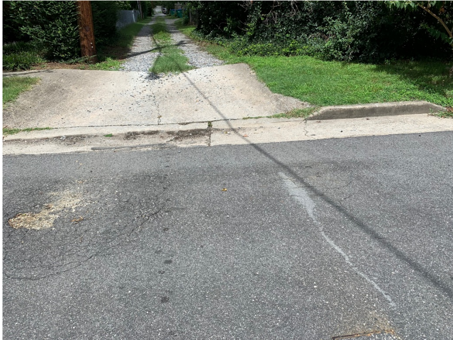
Cracking and depression near alley entrance
