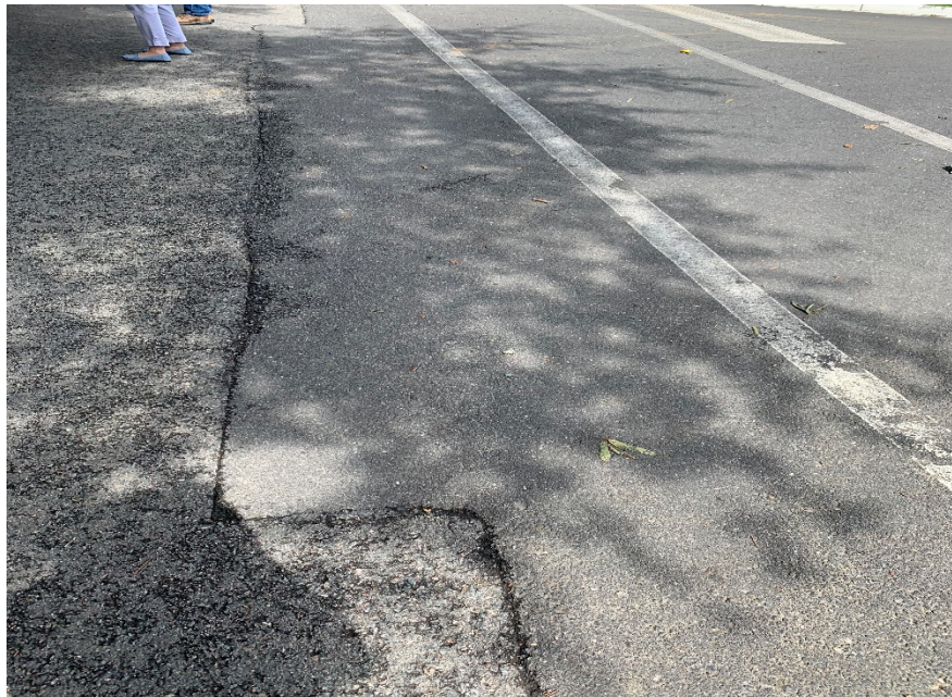
Fatigue and cracking
