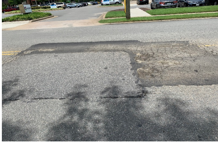
Multiple patches on top of each other
