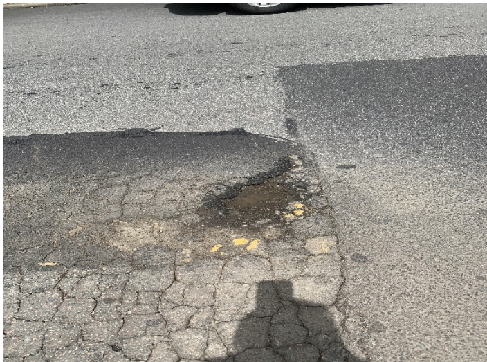
Cracking in a patch and standing water
