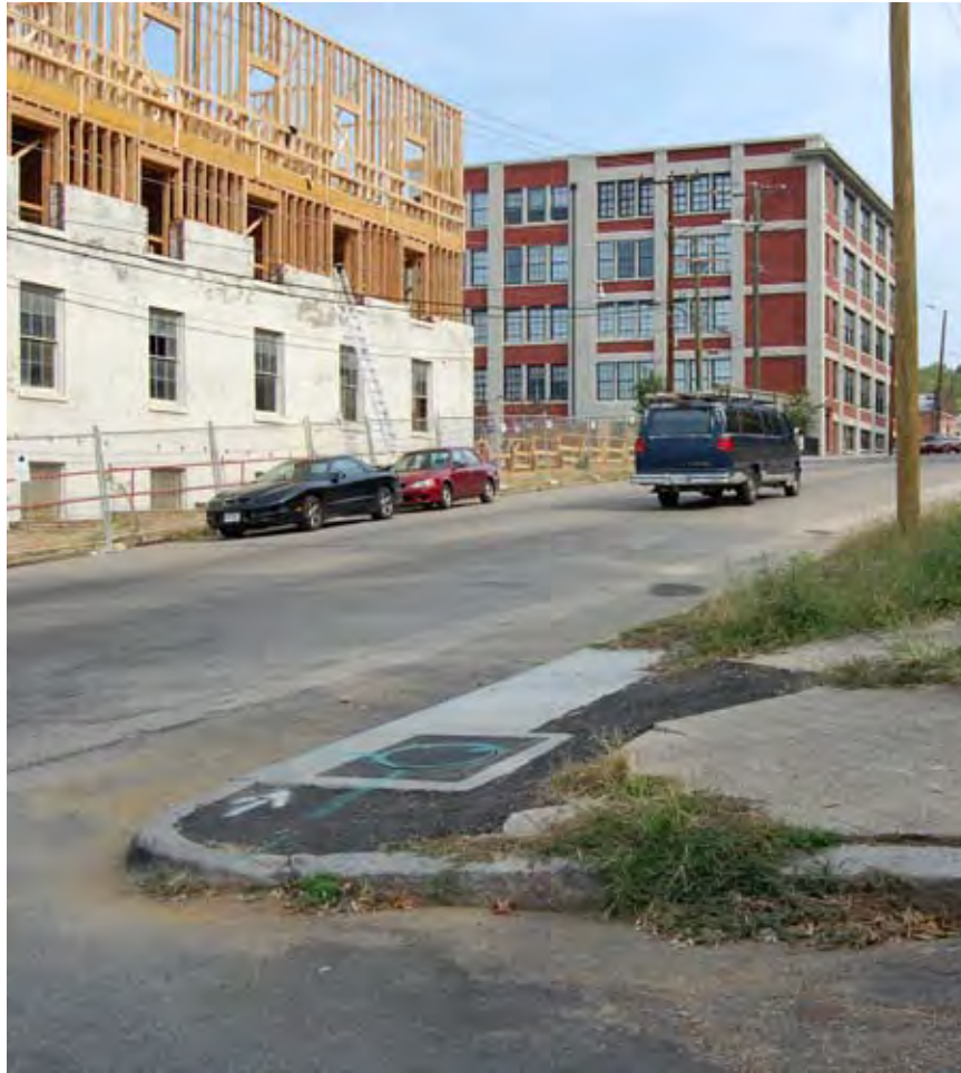
Broken and overgrown sidewalks in Shockoe impede pedestrian activity.
