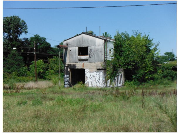
View of the former pump house looking northwest showing overhead electrical lines.
