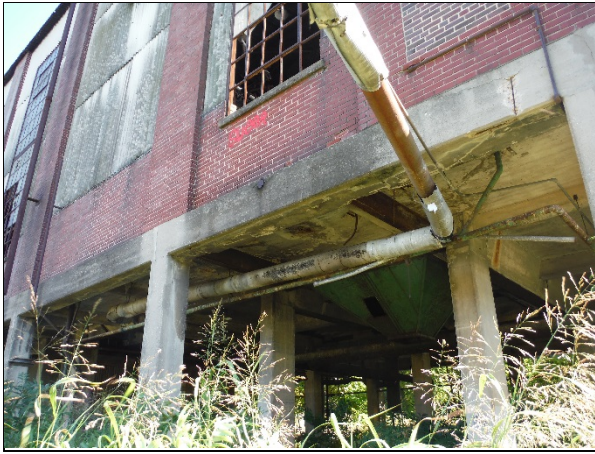
Lower portion of the former boiler room building showing elevated piping with suspected asbestos insulation.
