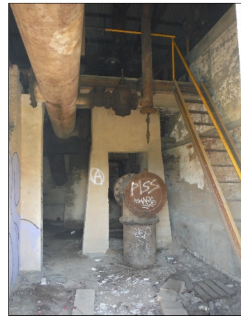
Interior of the engine room building showing ground pipes and valves.
