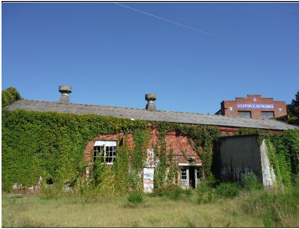
View of the southern face of the engine room building with the boiler room building beyond.
