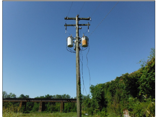
Pole mounted electrical transformers located to the southeast of the engine room building.
