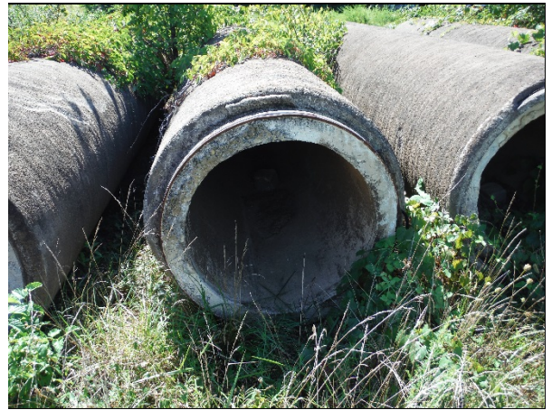
Concrete pipes located in the north central portion of the site suspected of containing asbestos.
