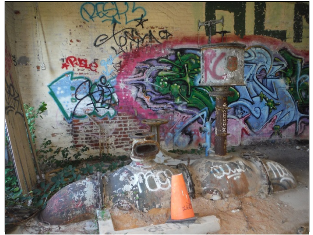
Interior of the engine room building showing partially buried pipes and valves.
