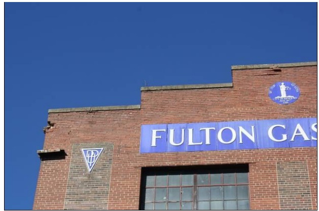
Figure 5-46. Detail of loose bricks.
