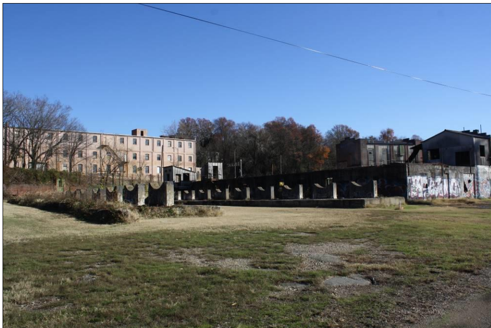
Figure 5-32. Building 3, Liquid Gas Condenser Tank supports, view northeast.
