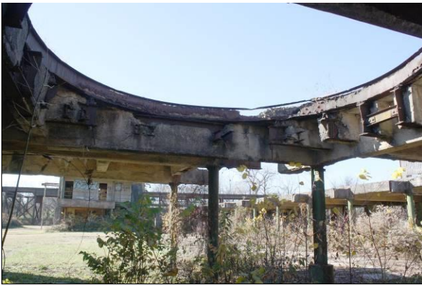
Figure 5-45. Detail of corroding concrete and steel.
