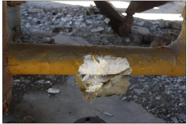
Figure 5-44. Detail of flaking asbestos.
