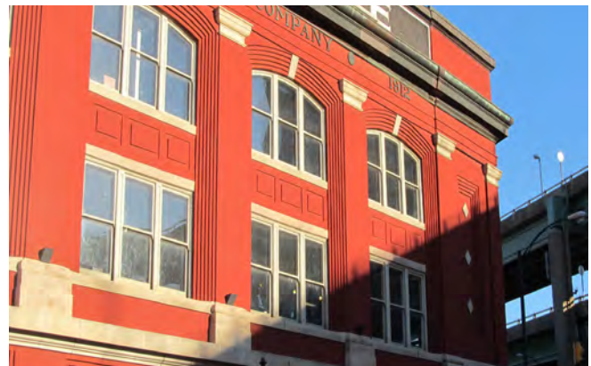
Detail -- Long facade organized vertically by pilasters and recessed wall plane containing symmetrically placed openings, decorative brickwork and stone accents.
